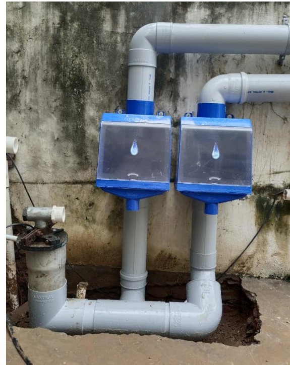
(b) Actual RWH system installed in a flat
